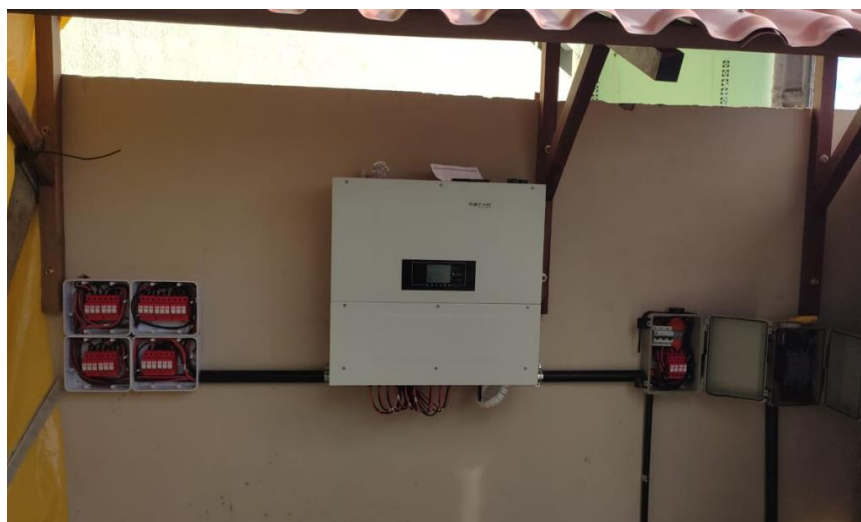
Figura 21: Inversor solar Sofar 50.000TL
