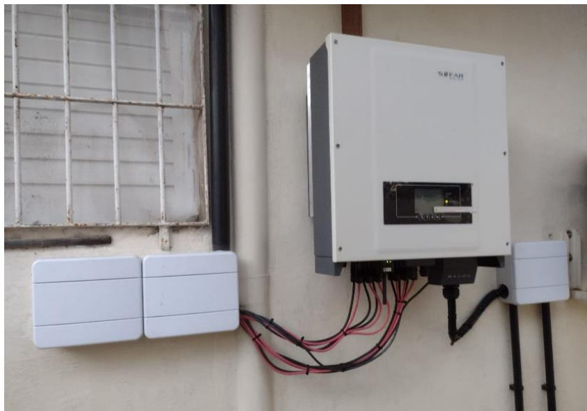
Figura 20: Inversor solar Sofar 30.000TL-G2
