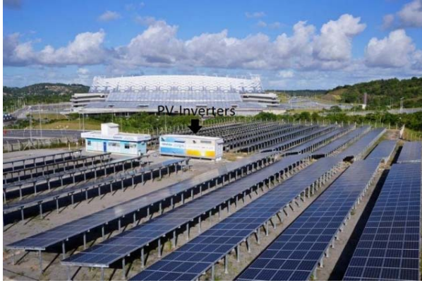
Fig. 1. Power Plant in São Lourenço da Mata – PE, Brazil.
